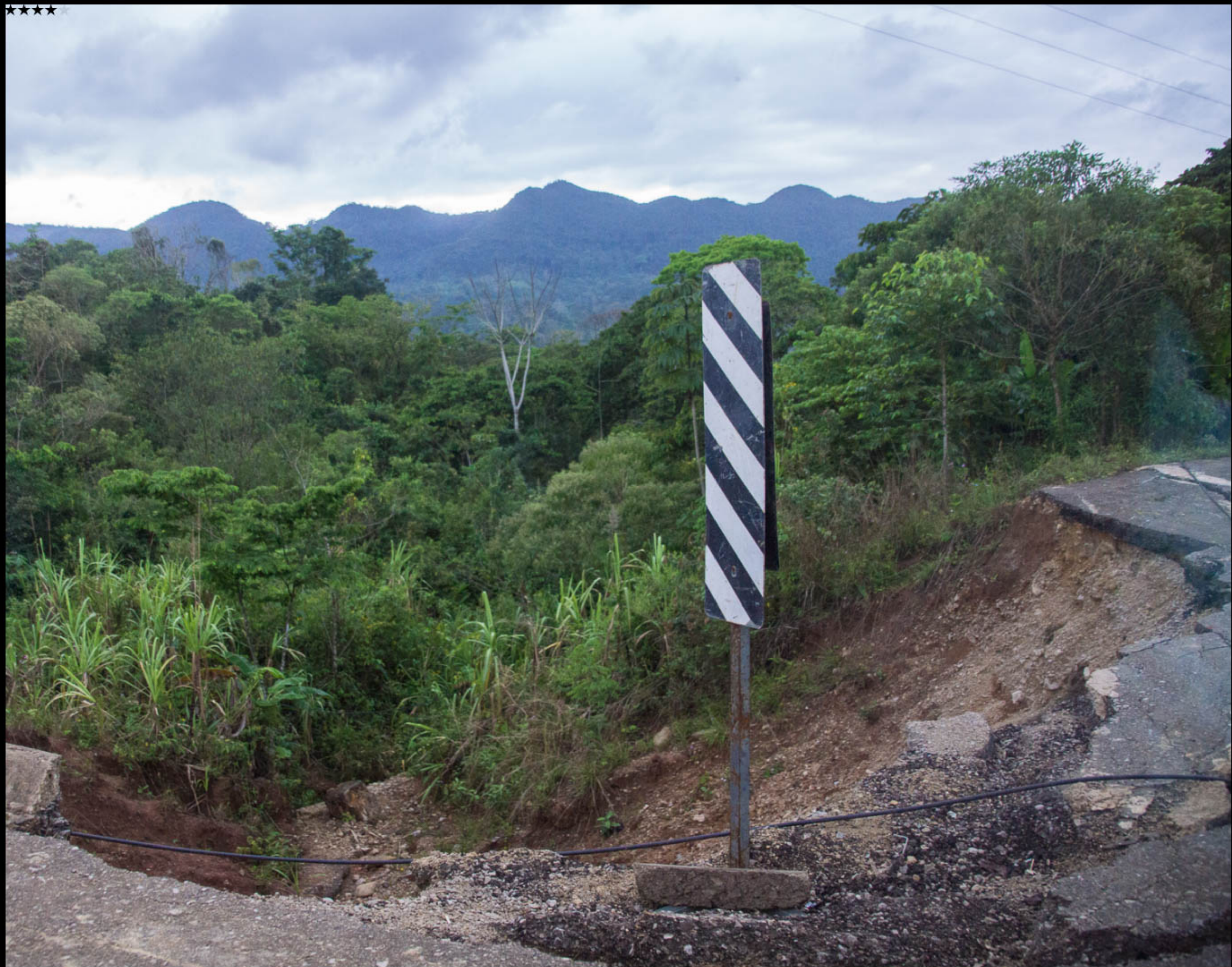
More road damage
