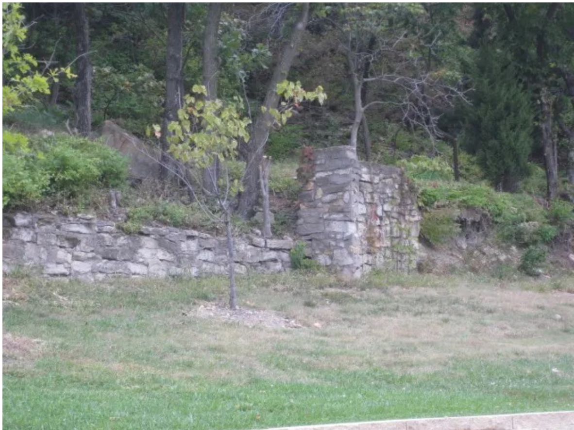
Hand Laid Rock Retaining wall, at this point the trail is above the wall
